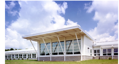
Shading devices are designed based on solar analysis. They should not block any views to the exterior.
